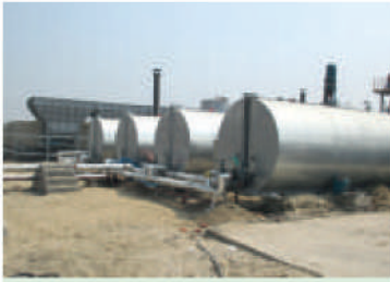
Storage Tank, Bangladesh
