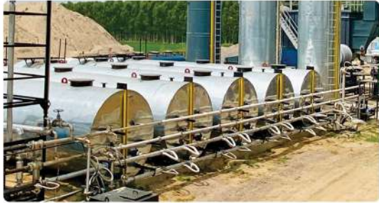
CYLINDRICAL BITUMEN TANK
