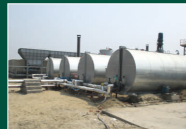
Storage tank, Bangladesh
